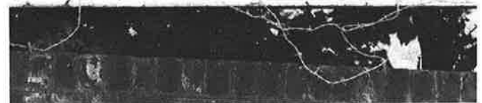
Closed and vandalised 1985
